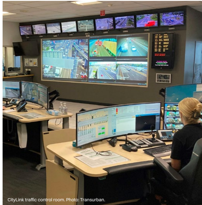
CityLink traffic control room. Photo: Transurban.
